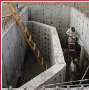
Junction Box - Towne Lake
