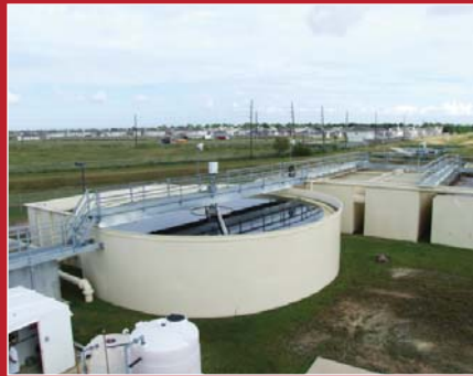
HC MUD No. 127 - WWTP
