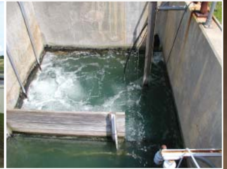
Williamsburg Regional - WWTP
